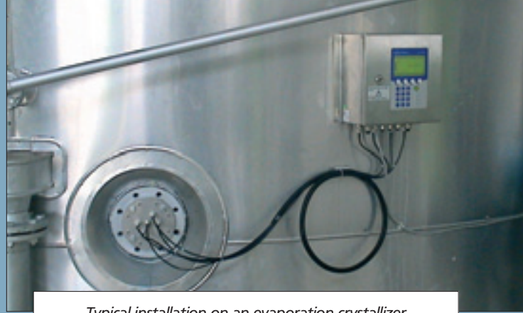
Typical installation on an evaporation crystallizer
